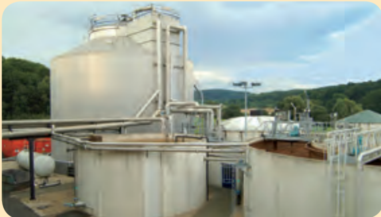
methane plant / production of energy / anaerobic
